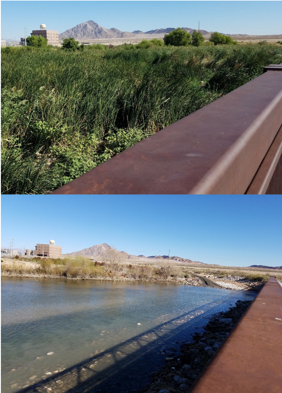
Figure 32. Before (top) and after (bottom) photographs of clearing of vegetation upstream of the Upper Diversion Weir and bridge.
