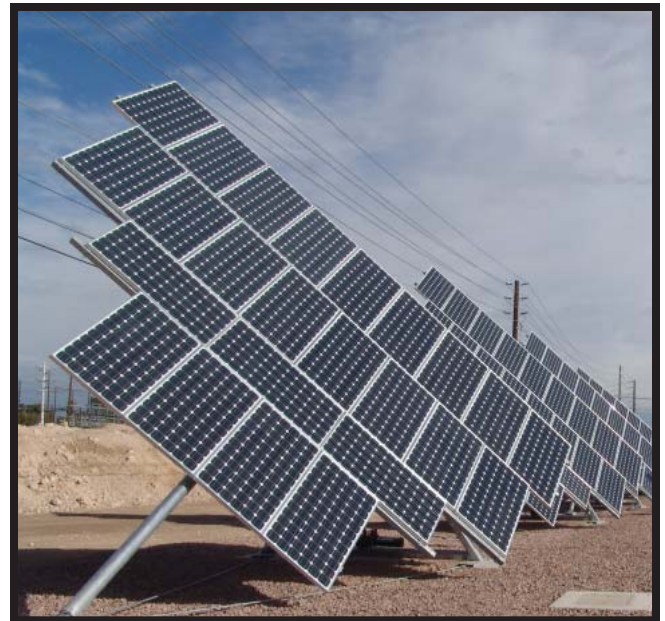
Solar panels at Las Vegas Valley Water District.
