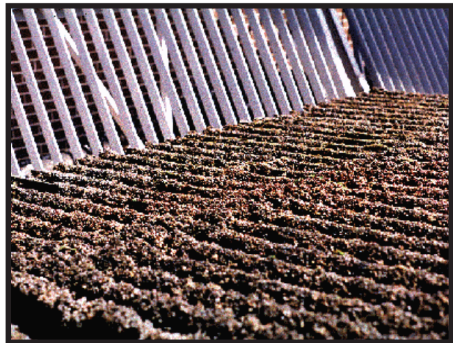
Quagga mussels clogging a grate.
