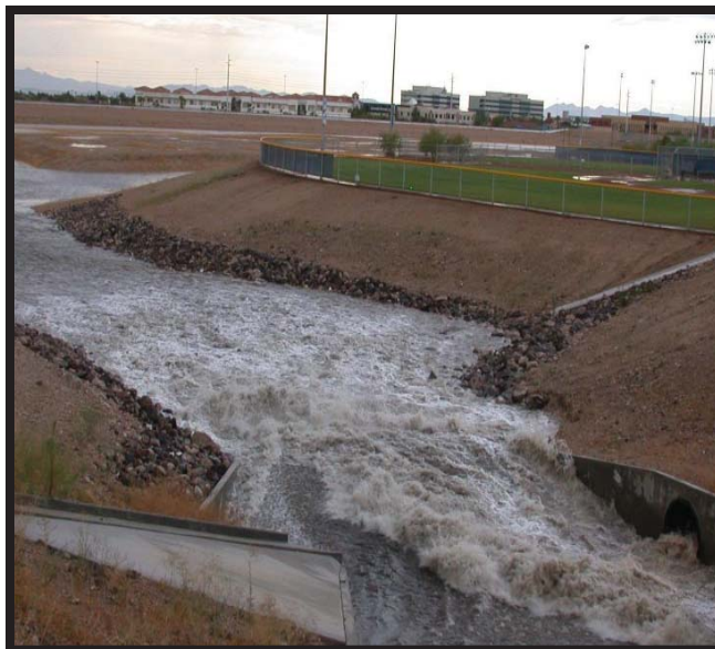
Stormwater detention basin at Doc Romeo Park, Las Vegas.
