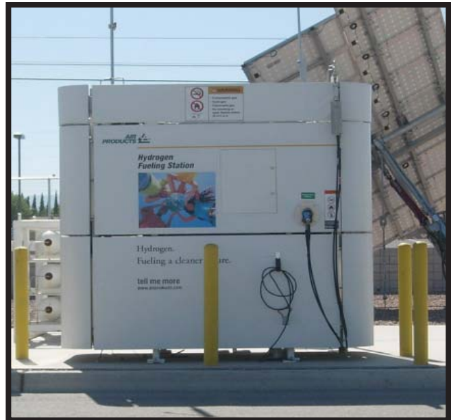
Hydrogen Fueling Station at Las Vegas Valley Water District.
