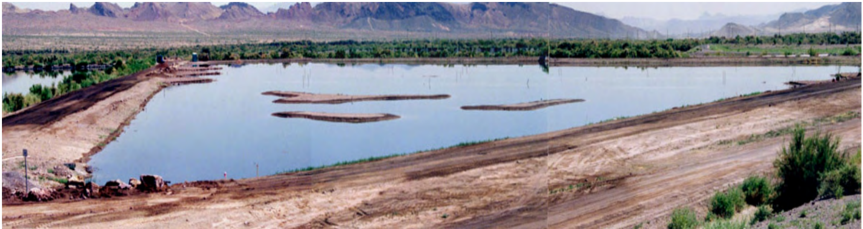
The Demonstration Wetland at COH after filling with treated wastewater. Photo was taken on May 9, 2001.
